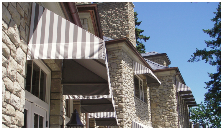
This stationary awning with closed-in sides provides nearly complete solar shading and only limits view of the sky.
